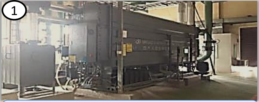
1 Utilization of Waste Heat by Installing VAM of 300 TR for Engine Assembly
